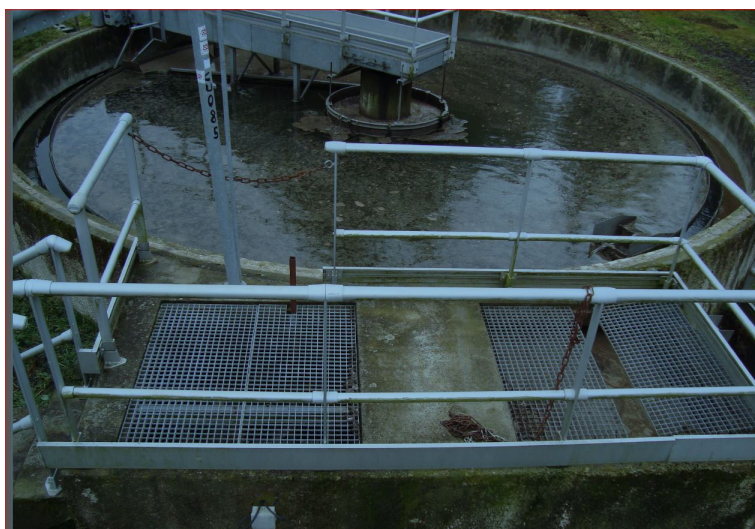
Clarificateur Station d'Epuration
